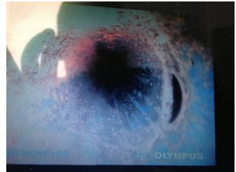
Video scope Images of Defective Tubes
