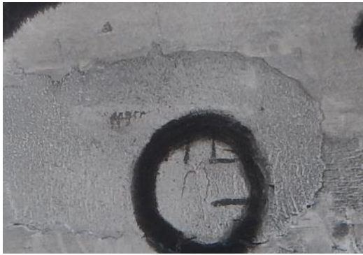
Fig 4: MPI defect signal
