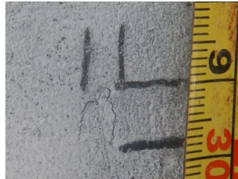
Fig 4: MPI defect signal with measurement
