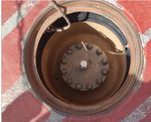
Fig.2 – Sensor location at Hydrant Valve
